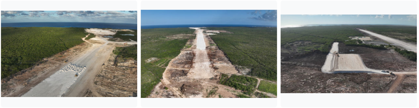
Real progress: Aerial views of the runway extension and apron construction at Deadman's Cay International Airport
